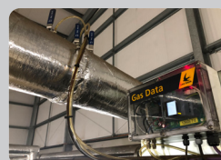
Gas Flow Monitoring
